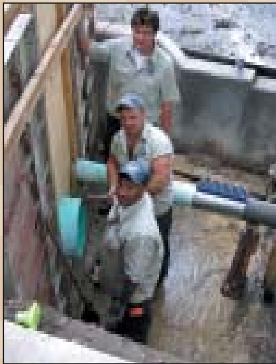
Staff from Public Works form a retaining wall at NE 5 th Avenue as a part of the Duckpond Restoration Project.
